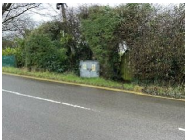
Figure 3 – existing control kiosk
