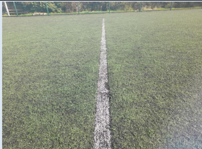
Damaged line markings
