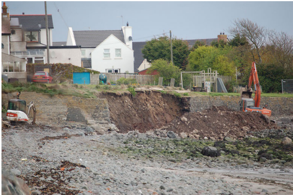
Removal and replacement of sea defences for Residential Property Ballyvester Beach – May 2010
