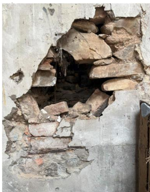
Figure 9: Photograph supplied by the agent of chimney flue
