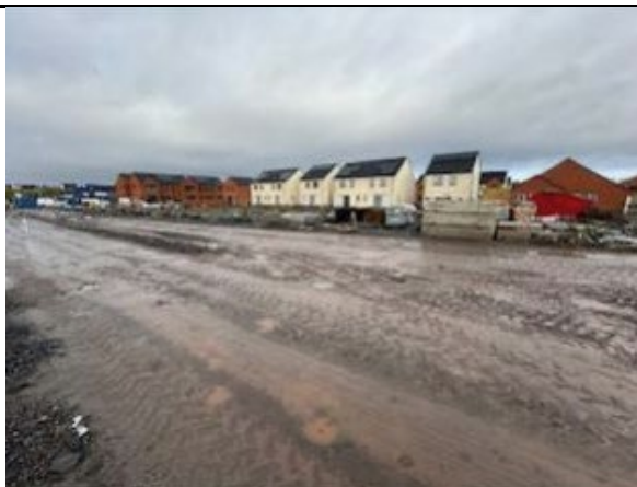
Figure 2 – view towards centre of site – some houses largely complete, with only foundations in place on houses to south
