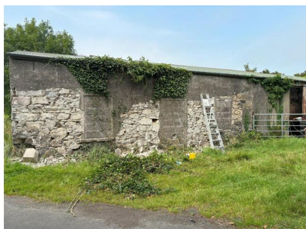
Figure 7: Photograph submitted by the agent to demonstrate removal of portions of render.
