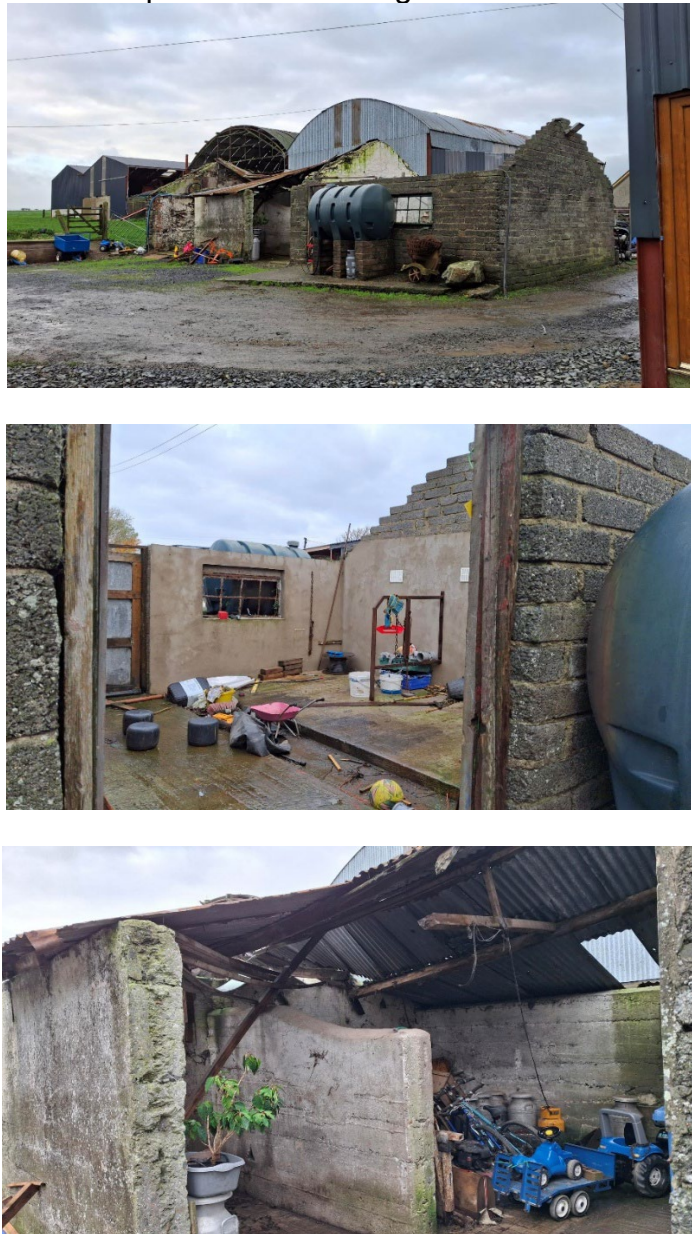
Figure 3 Photographs of the existing shed which is in a bad state of repair and is to be replaced by Structure B annotated on the site plan.
