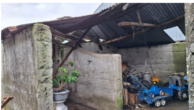
Figure B. Photos show the existing shed which is in a bad state of repair and is to be replaced by Structure B annotated on the site plan.
