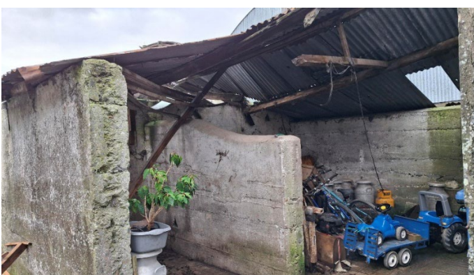
Figure 3 Photographs of the existing shed which is in a bad state of repair and is to be replaced by Structure B annotated on the site plan.
