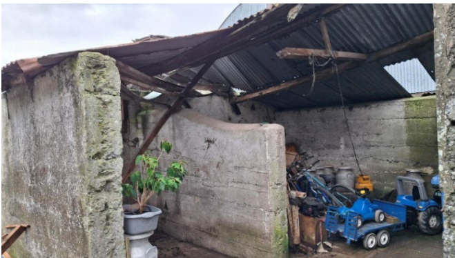
Figure B. Photos show the existing shed which is in a bad state of repair and is to be replaced by Structure B annotated on the site plan.
