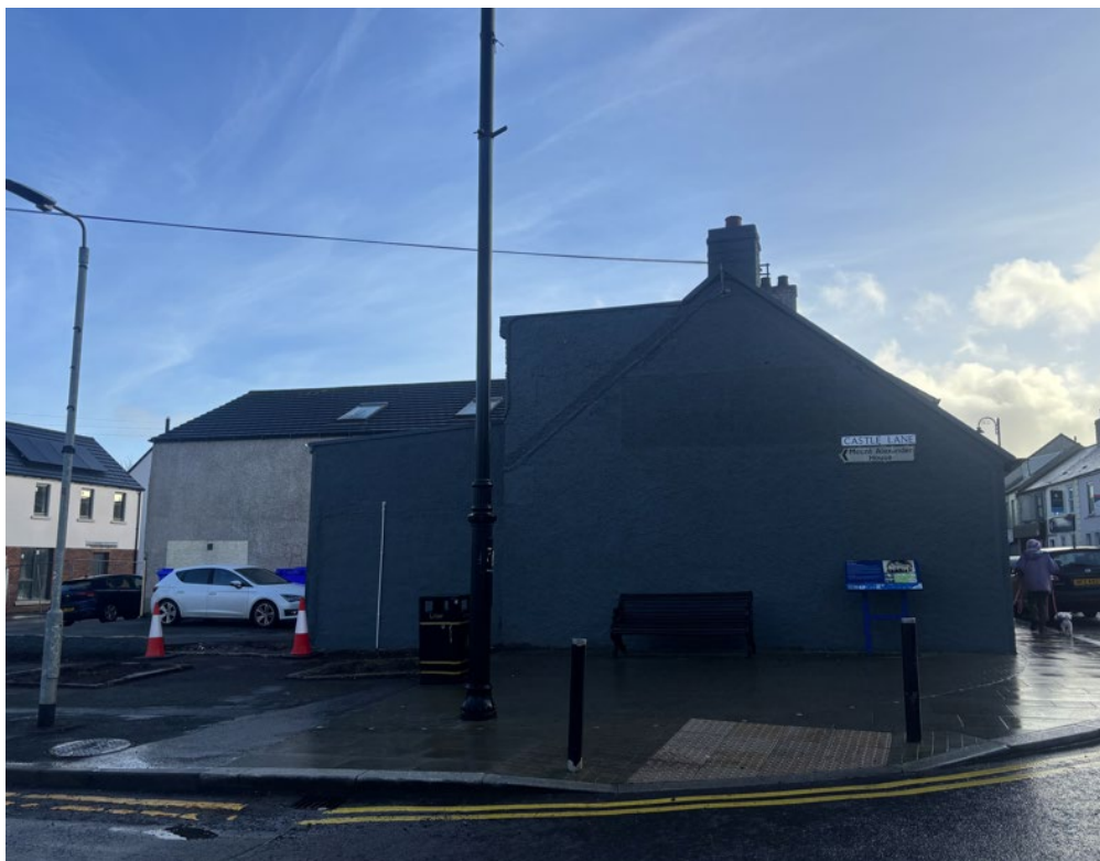
Retrospective works carried out to rear of building – increase in height to return and new steel clad finishes
