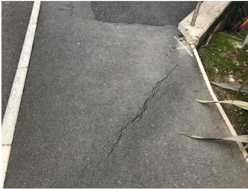
e) Uneven, cracked footways at southern car park entrance path.
