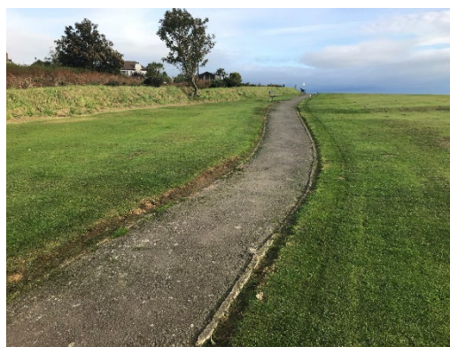
d) Uneven narrow footways and grass encroachment on upper path.
