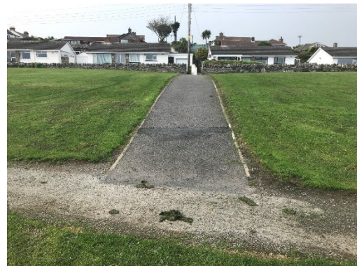
j) Steep gradient path from Marine Drive and weathered loose gravel on connecting path.
