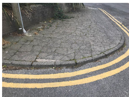
o) Broken footways on Railway Street and no tactile paving, unsuitable for wheelchair users.
