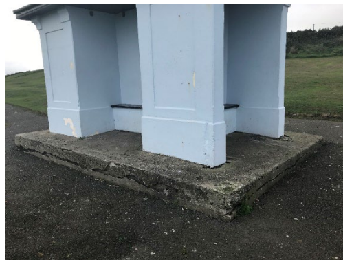
l) Poorly maintained shelters unsuitable for wheelchair users due to ground levels.
