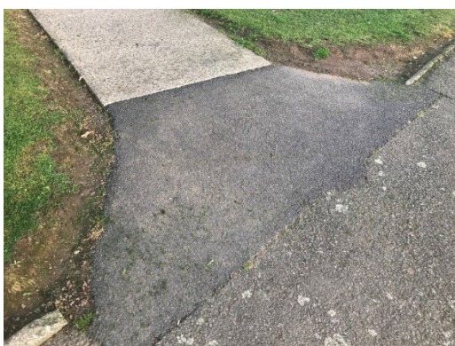
a) Inconsistent materials, steep gradient and low-quality repair to path at Millisle Road pedestrian access.
