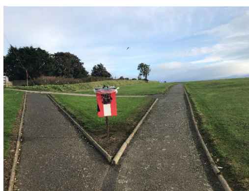
b) Inconsistent edging materials and steep gradient at Milisle Road pedestrian access.
