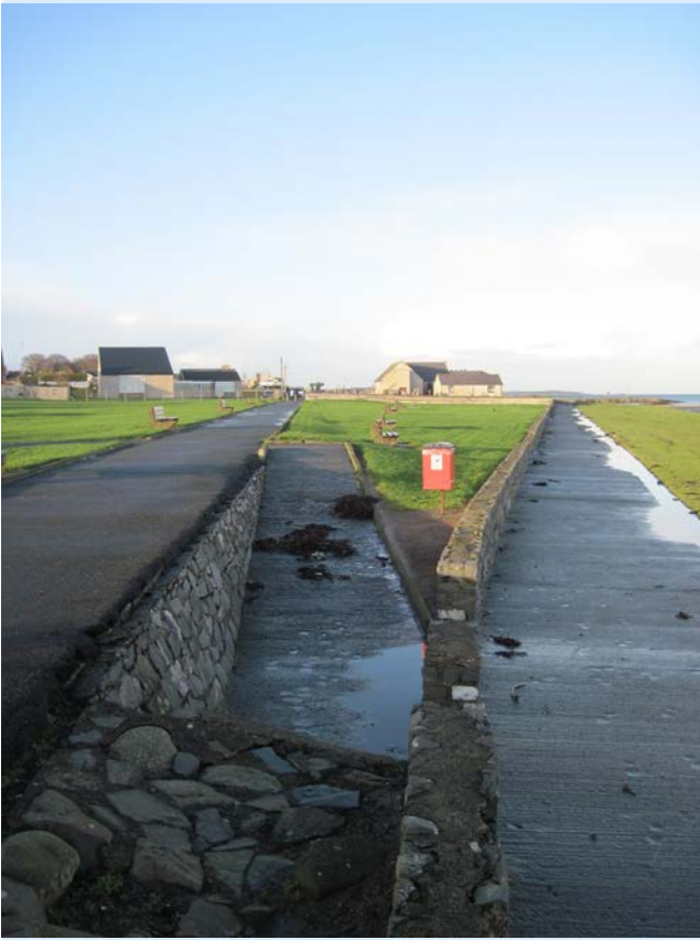
Paths and ramps - surface upgrade needed
